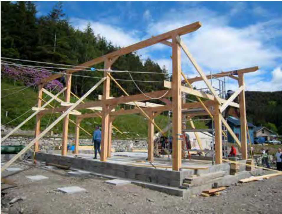
A home-grown Douglas fir house frame under construction in Wester Ross by Alba Green Oak Frames.
