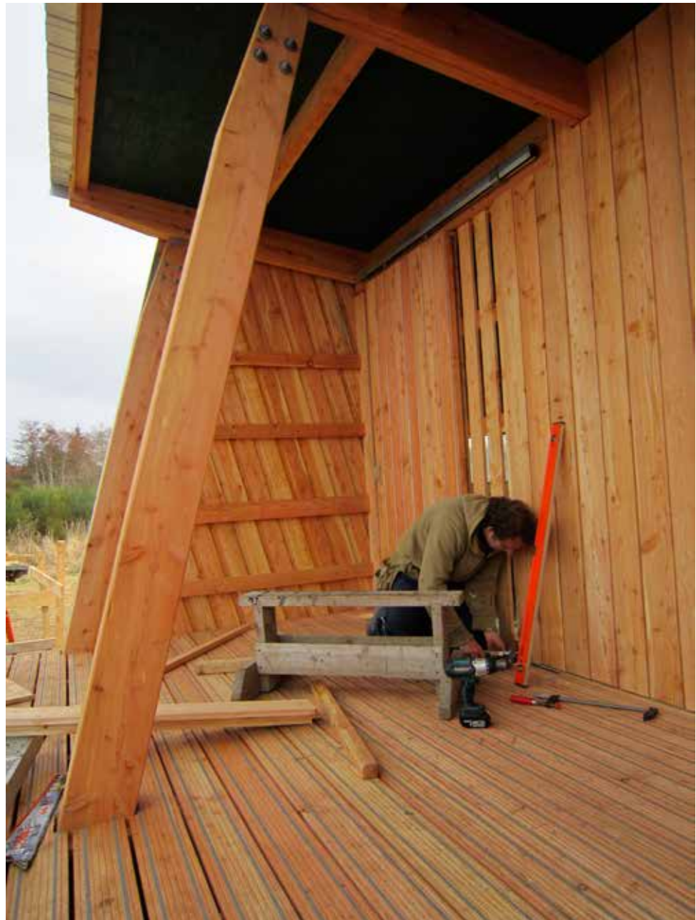
A building made entirely out of Highland-grown European larch: post and beam frame, cladding and decking.
