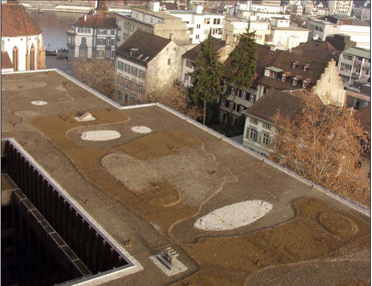
Figure 2: Newly constructed green roof on the Klinikum 2 of the Cantonal Hospital of Basel, built in accordance with the city's new guidelines on green roofs and urban biodiversity. (Photo: Stephan Brenneisen)
