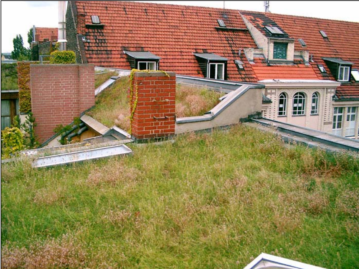
Figure 1b: The PLU research site in Berlin-Kreuzberg. In the foreground is a portion of flat sub-roof 1, with Allium species in fruit. In the background, the 47-degree pitched sub-roof 2 is visible.
