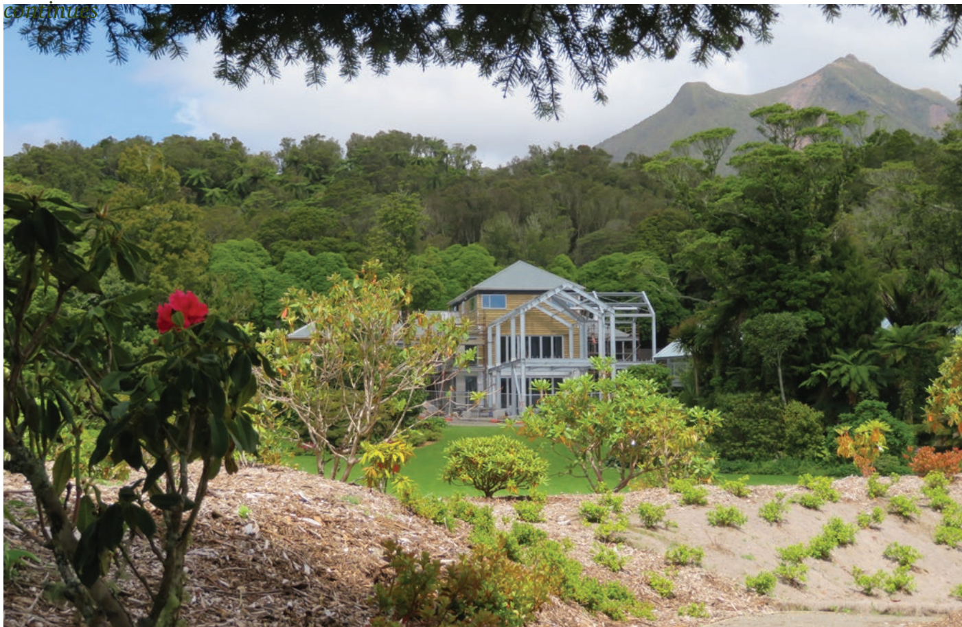
The Rainforest Pavillion under construction (the Gatehouse upgraded) from the Misty Knoll.
