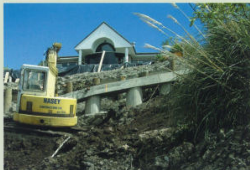
A reinforced concrete palisade wall is being constructed several metres inland of the cliff edge.
