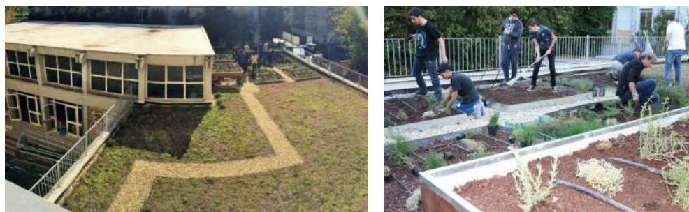
Fig.1. Experimental green roof. [a] General view, [b] installation made with the collaboration of the students
