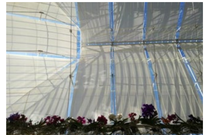
Figure 5: Automated ceiling screens
