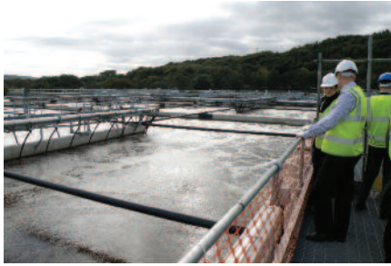
Utility assets – at the heart of the benchmarking of management and operations (picture taken during site visit to Yorkshire Water's Esholt wastewater treatment plant (UK) during the European Benchmarking Co-operation 2009 benchmarking exercise).
