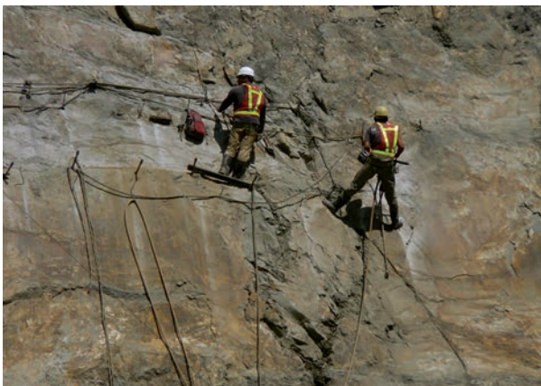
Photo 11/ “Mountain plumbing”, to distribute the flow of water and prevent it from cascading in concentrated areas.
