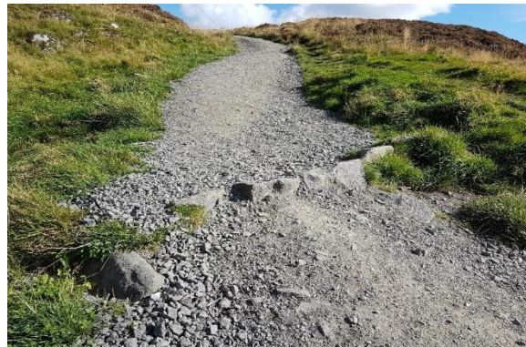
Fig 6. A water bar blocked with surface aggregate after heavy rain.
