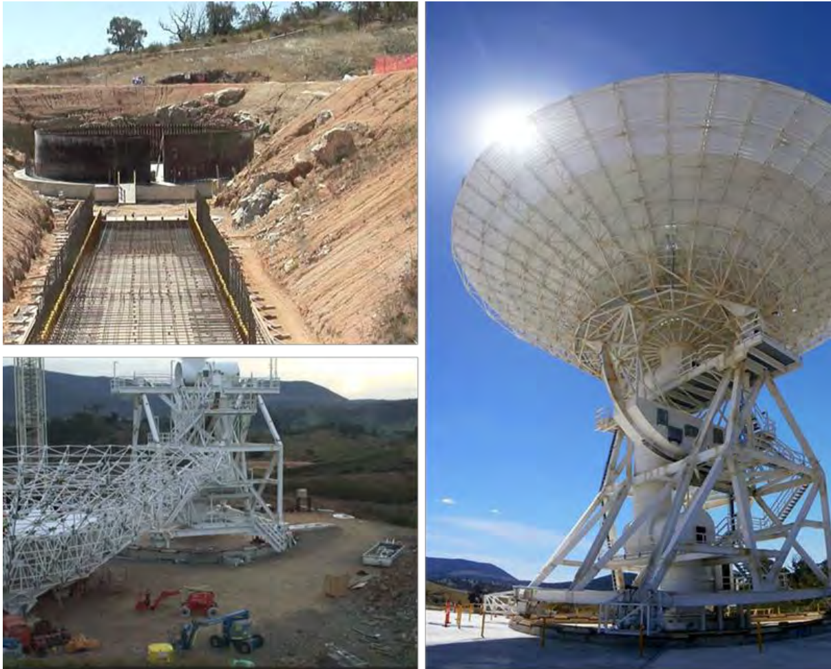
Figure 2-5: Deep Space Navigation (DSN) Antenna, up to 45m.
