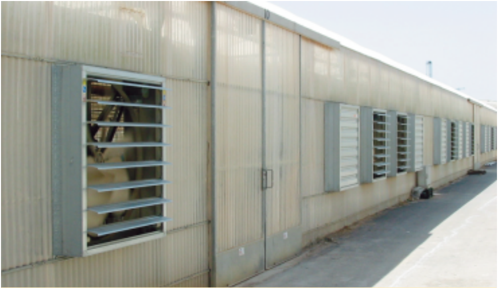
Extractores exteriores de cooling system.
