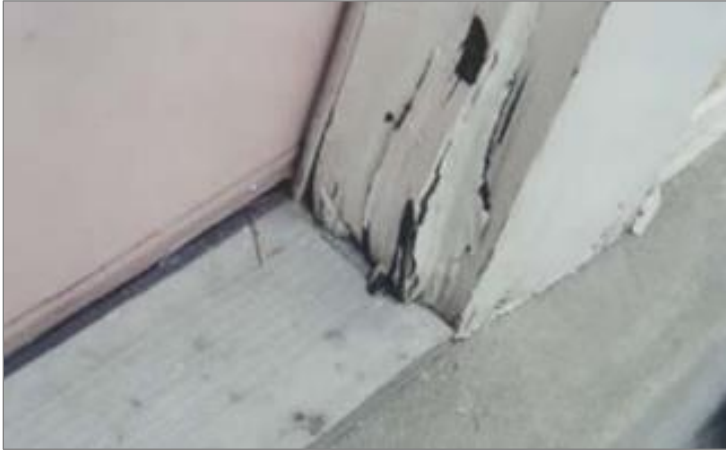
Figure 28. Rotted door frame (Division of Agriculture and Natural Resources).
