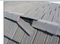
Figure 7. Displaced tiles allow ember entry (FEMA, 2008a)
