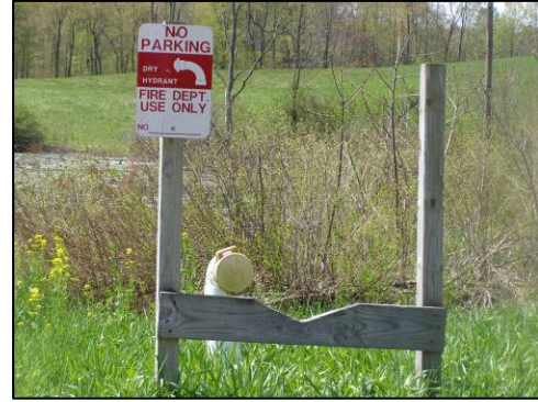
Dry hydrants provide water for use during emergencies in areas where no public water system is available
