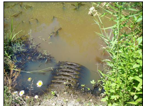
Culverts are used to control the movement of stormwater under roadways and through urbanized areas
