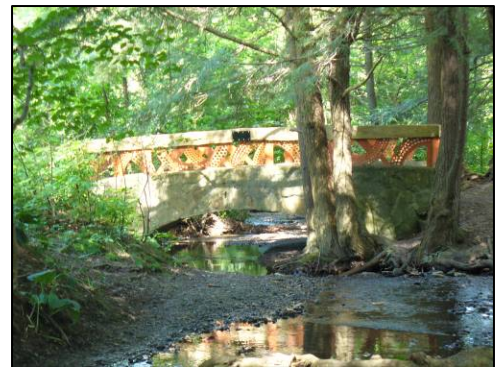
Along Bear Creek, erosion is noticeable
