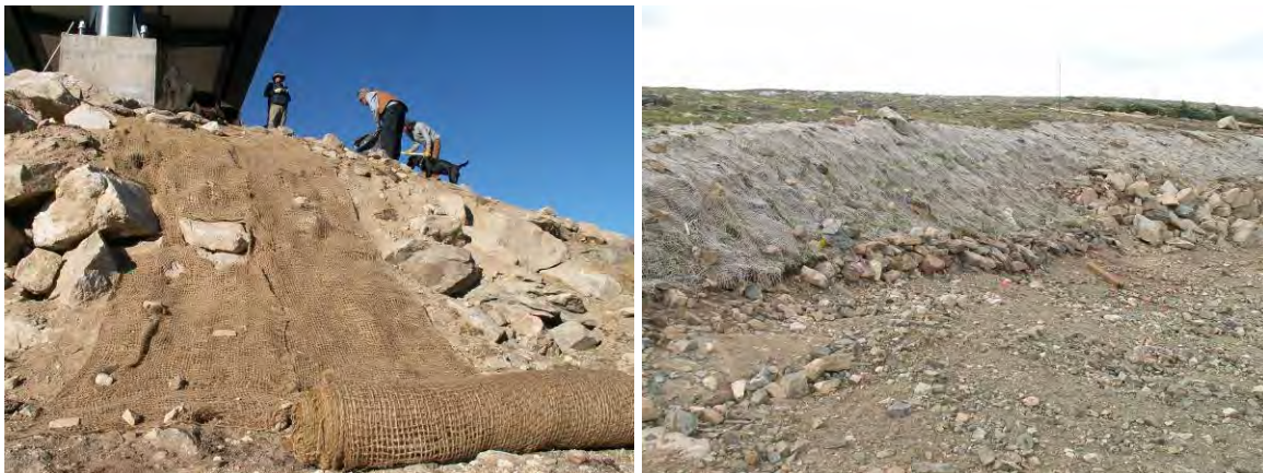
Photo: Jute mat installation Panoramic lift. (Right) Jute mat installation Eagle Wind lift
