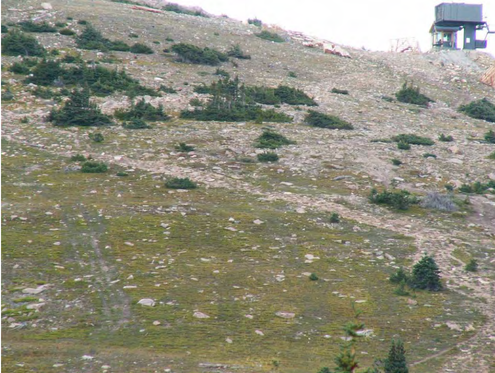
Photo: Utility trench disturbance 1st year blending completely at the upper portion and well in the center of photo
