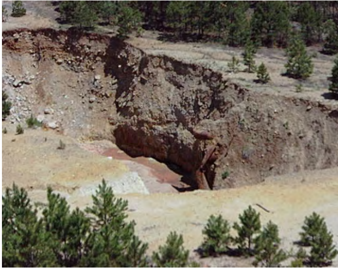
Photo 5. Interception of Balarat Gulch by largest subsidence pit.
