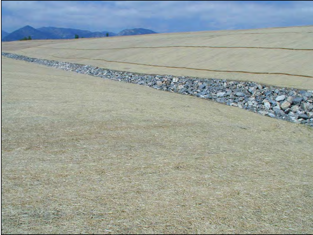
Figure 3. Temporary erosion blankets (and wattles on far hillside) used to protect soil and prevent erosion on the hillslopes at the Site.
