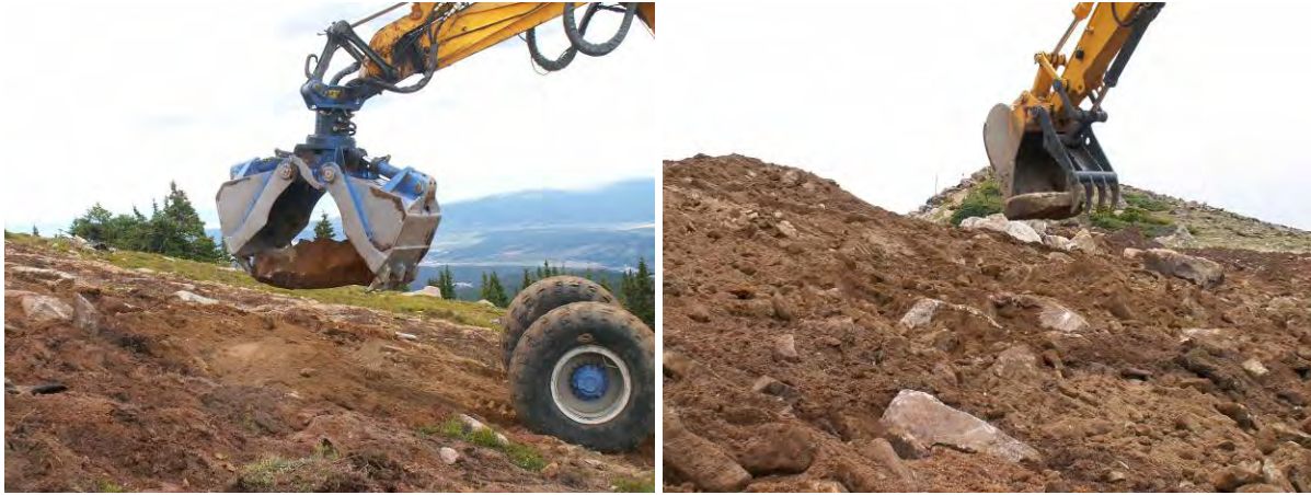
Photo: Eagle Wind rock placement with clam bucket and spider hoe. (Right) Panoramic lift rock placement with excavator with a bucket thumb
