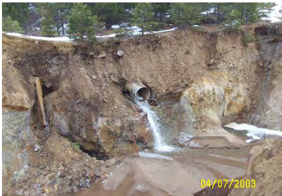
Photo 7. Subsidence pit intercepting Balarat Gulch.
