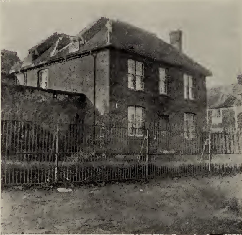
Chimneys of House at Writtle (see p. 140) broken off at bases and laid down intact on sloping roof.
