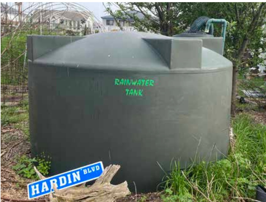
1 of 2 water tanks
