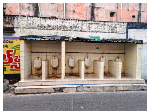
Figure B: unhygienic condition of Urinals
