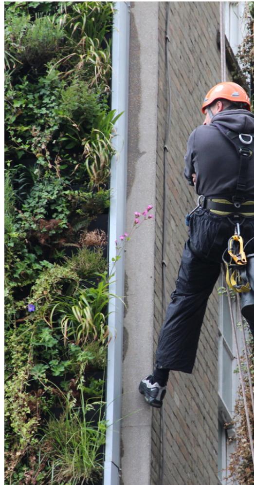
Living Wall System maintenance Photo: Maria Ignatieva
