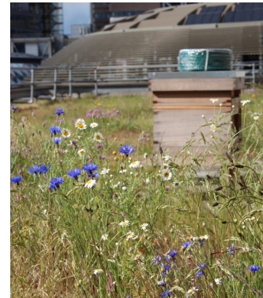
An extensive green roof with meadow, Sedum plants and bee hives Photo: Maria Ignatieva
