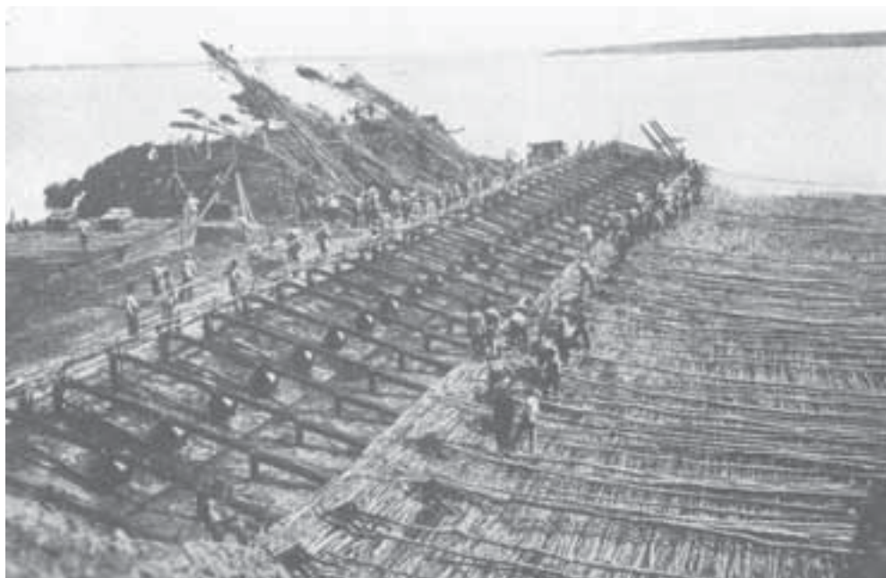
Fig. 6.8. Construction of black willow mats in 1915 for riverbank stabilization in the LMAV. Photo courtesy of J. Stanturf.
