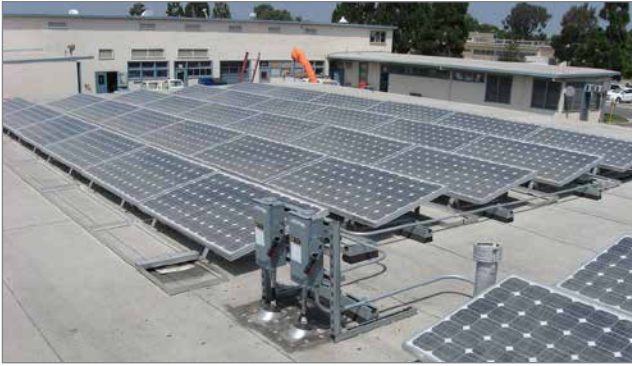
Figure 4.13 B. Example of rooftop solar installation.
