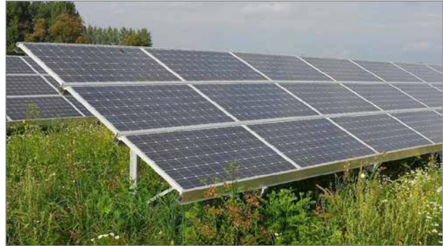
Figure 4.13 A. Example of a large scale solar energy system.
