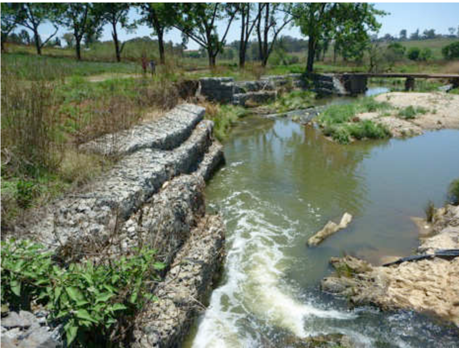
Figure 42 Eroded bank of the Jukskei River and collapsing gabion structures
