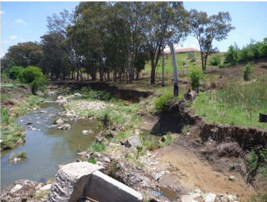
Figure 44 Eroded bank of the Jukskei River and collapsed concrete structures
