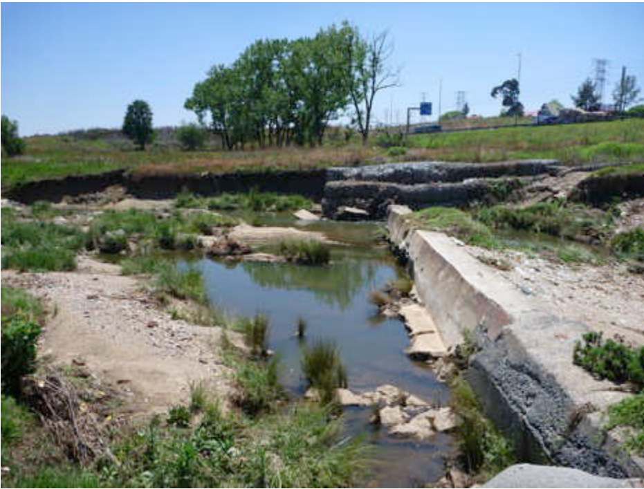
Figure 43 Collapsing gabion structures and a silted-up weir
