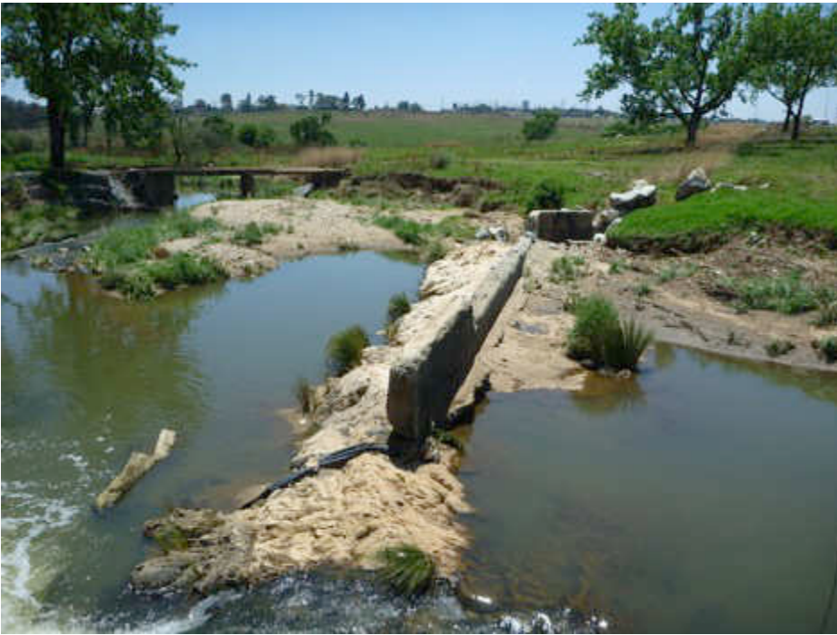
Figure 41 Eroded banks of the Jukskei River and a compromised weir
