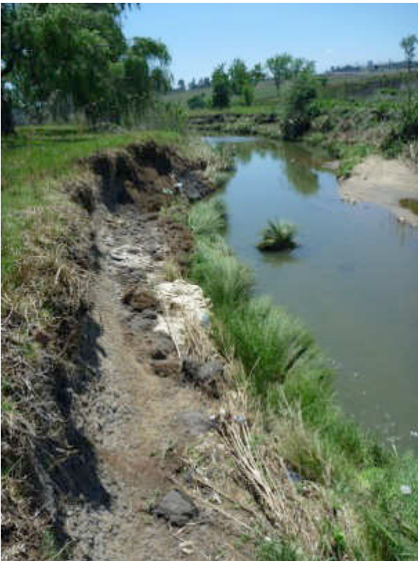
Figure 36 Eroded bank of the Jukskei River exhibiting soils that formed under uneroded valley bottom conditions
