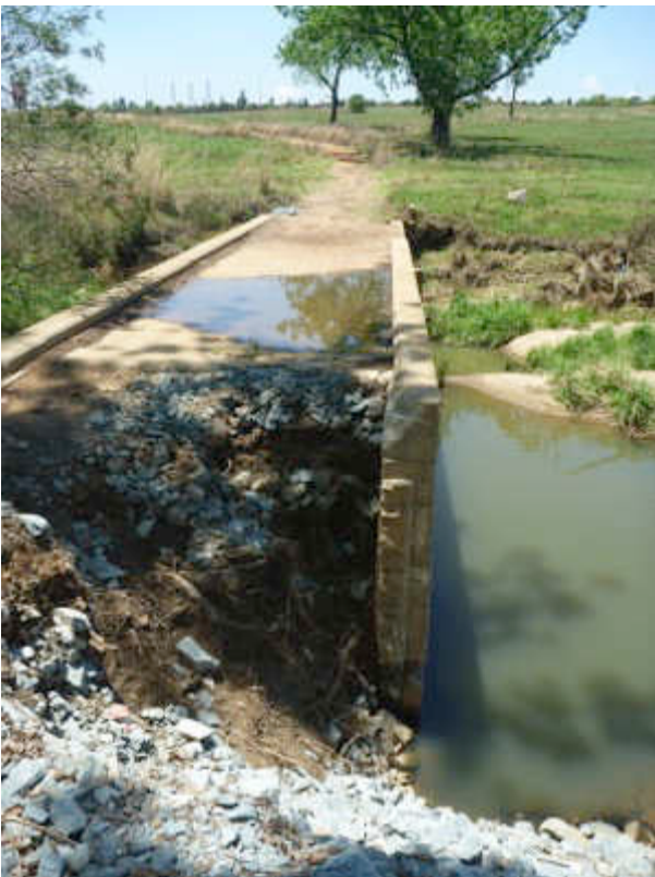
Figure 40 Eroded bank and compromised bridge (with signs of haphazard attempts at repair)
