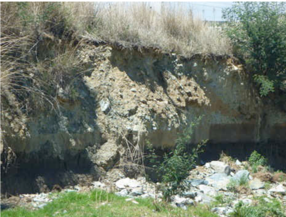
Figure 38 Eroded bank of the Jukskei River as a result of human activities
