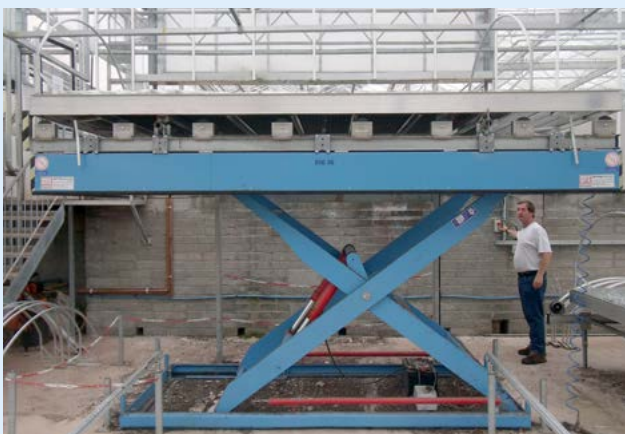
A mechanical lift allows benches to be moved between two levels
