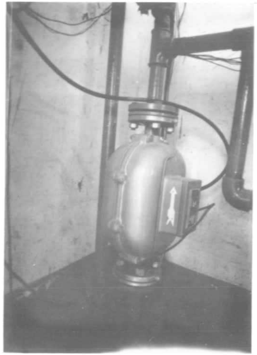
Plate 15. Electromagnetic flow meter (Photograph Pei Tiefan)
