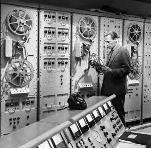
Fig. 2.91: Perfo tape machines in the control room of the Philips Pavilion: the two three-channel units for the music at left and one of the two fifteen-channel units for the control signals at right (the second is not visible in the photo). During performances, only one three-channel and one fifteen-channel machine were used at a time.
