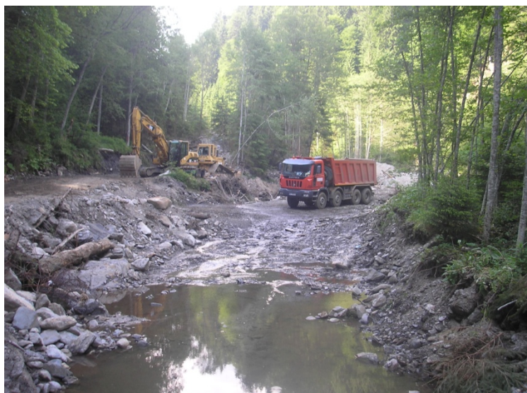
Figure 25: Heavy construction equipment work near the sampling station 13; lotic habitat negatively affected by works for Capra V micro hydro-power plant.
