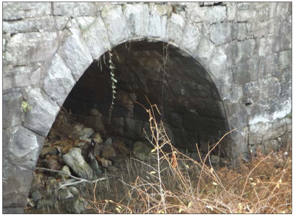
About halfway down the section between Route 169 and Golden Greek, the railbed passes over this historic arch bridge.
