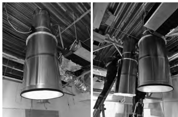
Fig.7. HLC “Solar LED-S” in the “Meeting room “ (installation process). ALB is located in the space of the technical floor, located above the ceiling of the “Meeting room” under the roof (internal design)
