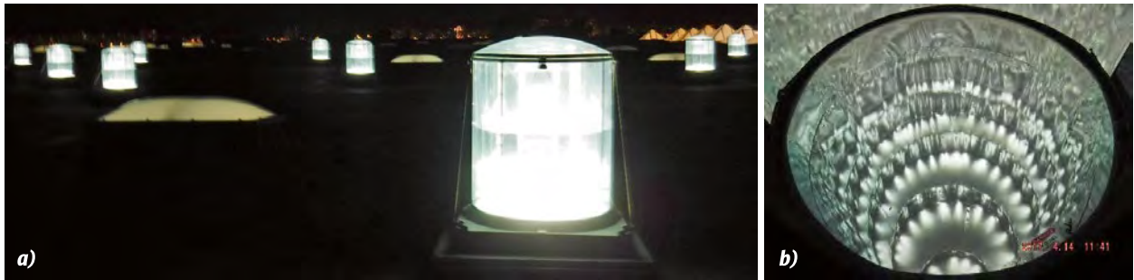
Fig.1. The illumination manifold as a result of “selling” reflections of the LED module luminous flux (a) and mirror reflection LED module (top view through a manifold in the channel of hollow tubular light guide) (b)
