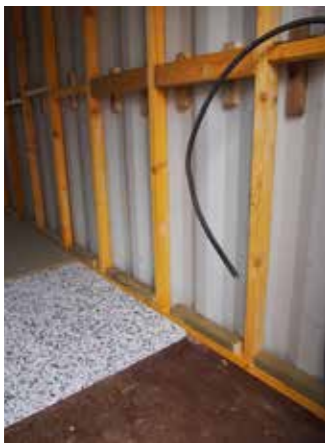
Drew fits out the container. The wooden frame will be insulated, and insulation is also laid between the original hardwood floor and a new floor.
