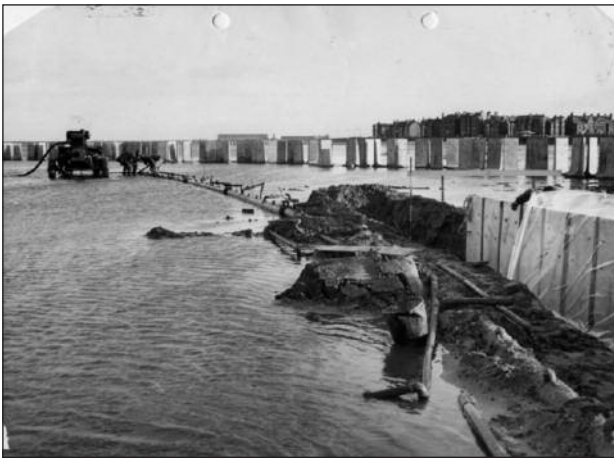
Plate 4. Photograph of construction of Marine Lake extension, with ground being dewatered during building of perimeter wall, looking west, with the Promenade in the background, dated 13th January 1962. (Image held in SMBC archive).
