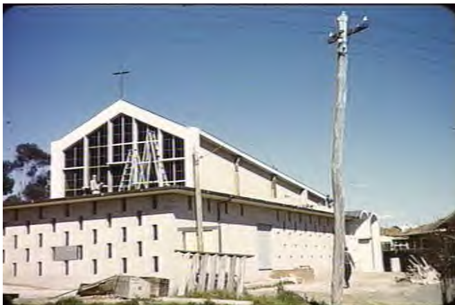
View to frontage and along west elevation, during construction (Source: Peter Wille, undated, SLV, no a22359)
