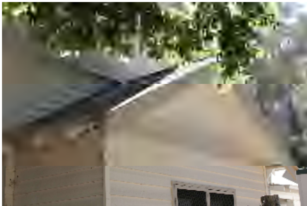
The gable end and roof form of the porch are likely original
