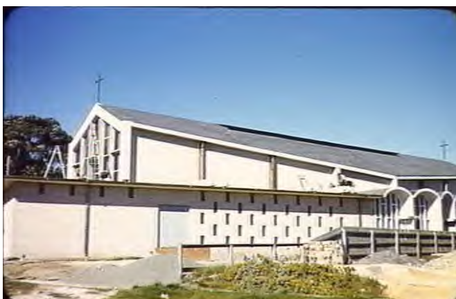
View to west elevation, during construction – note barrel vaulting (Source: Peter Wille, undated, SLV, no a22359)
