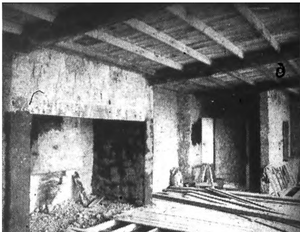
'Roof and floor construction shows in this progress shot.' (Source: Johnston, 'Built from the good earth', AHB June 1948, p29)
