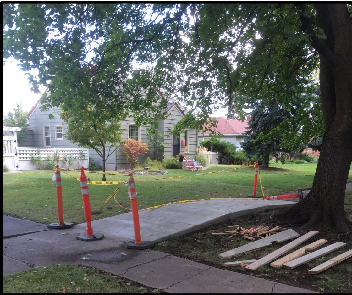
Sidewalk ramping raises the sidewalk over the root system.
