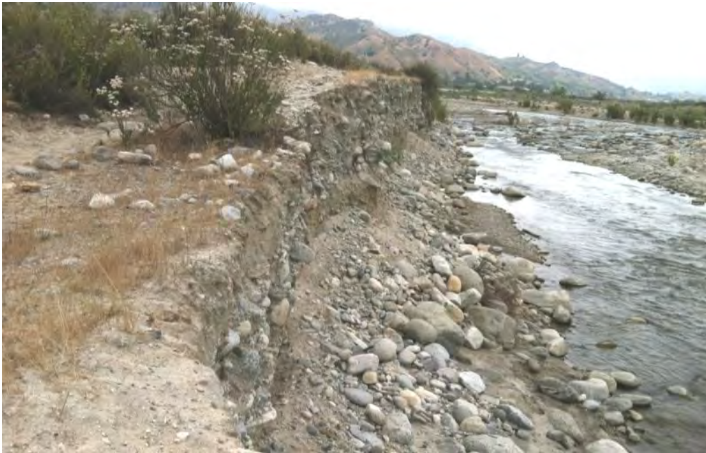
Figure 2. Site of trail erosion is the result of undercutting during high water flow periods. The horse trail is approximately 10 feet above the Wash.
