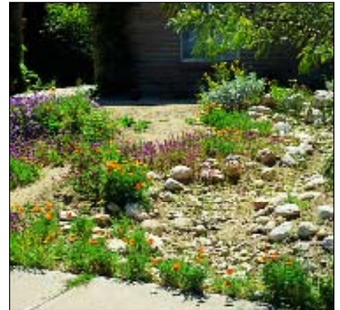
December: Time to do the heavy work, such as installing a dry creek bed for landscape interest and drainage.
