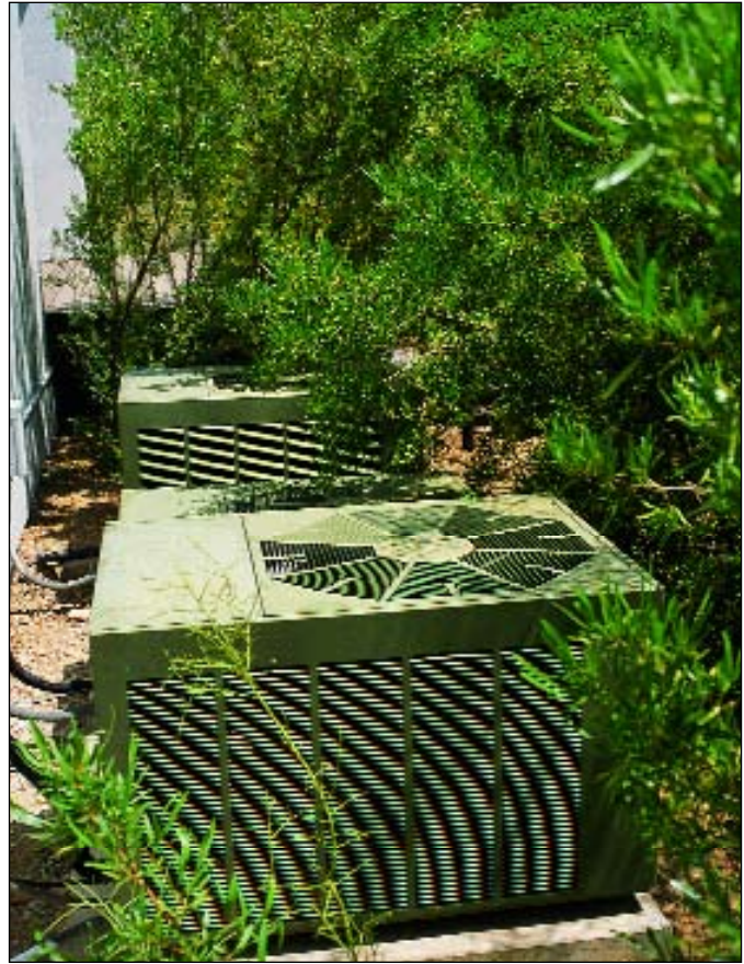
Shading air-conditioning units can reduce their workload, making them more energy-efficient.
