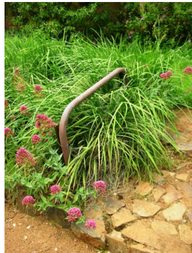
V20: Existing intrusive handrail needs to be replaced.
