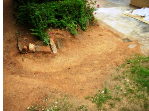
F38: Runoff near the gravel drive needs monitoring and the drain cleared.
