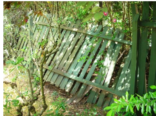
V16: One of the 1980's lapped fences (N/W) in need of repair.
