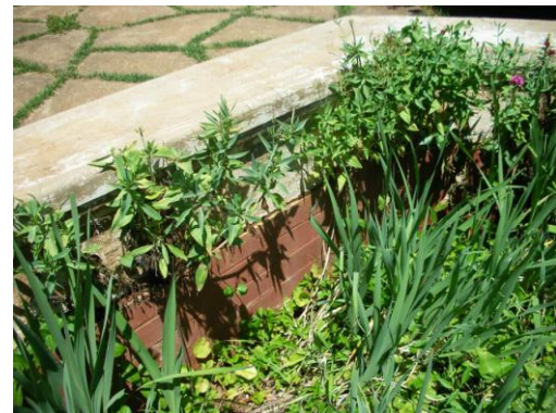
V18: Invasive SSP should be removed from entry wall.
