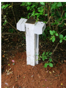
Figure 48: Intrusive Electrical Installation
