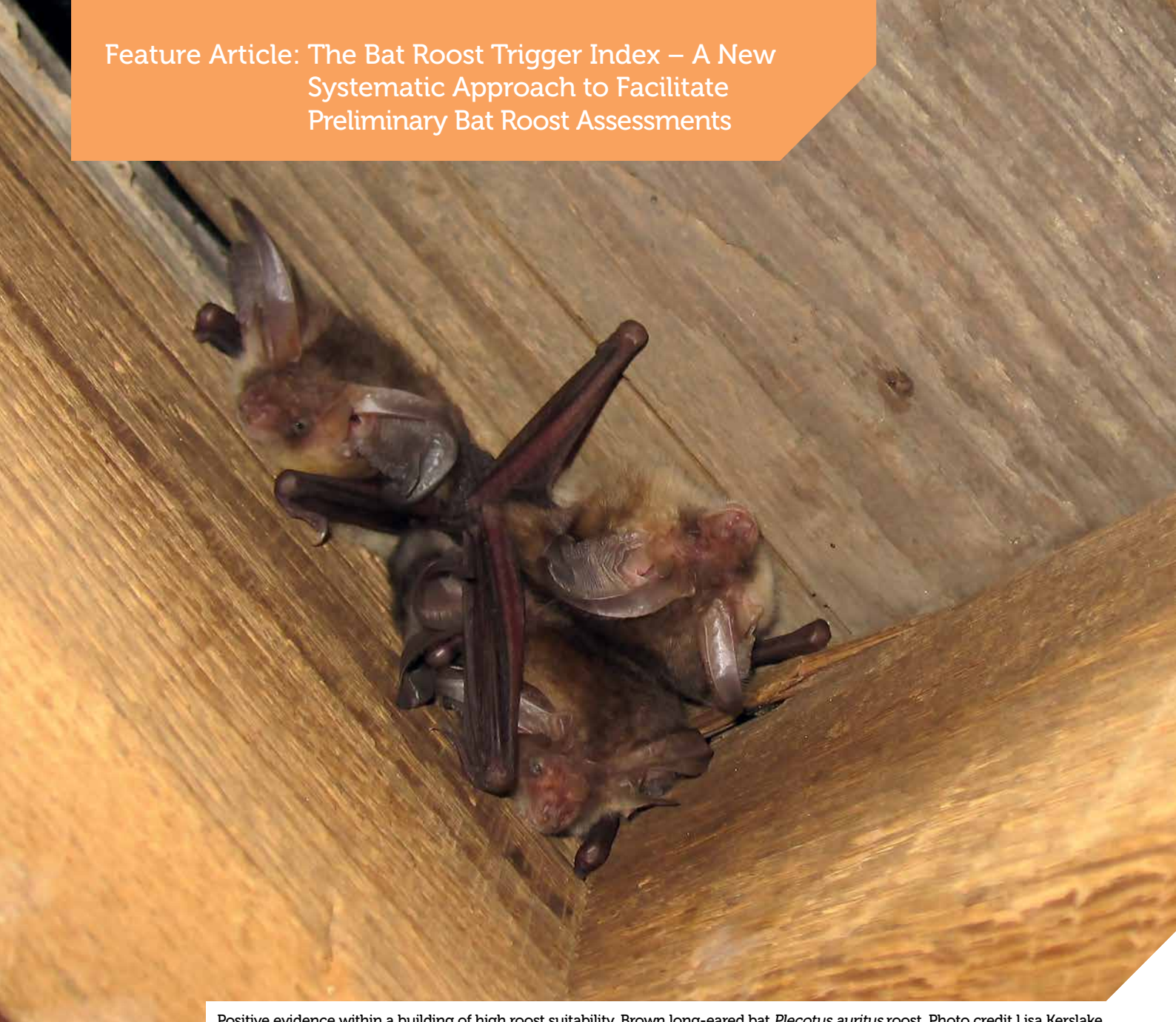
Positive evidence within a building of high roost suitability. Brown long-eared bat Plecotus auritus roost. Photo credit Lisa Kerslake.
