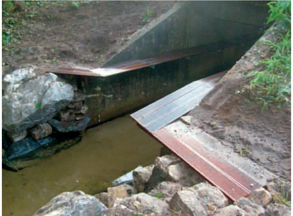
Figure 5. Another example of a specific mink culvert correctly adjusted to the ground level.
