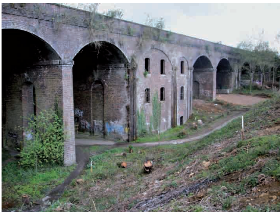
Figure 3. The railway viaduct and former dye-works at the Capels Mill site adjacent to the route of the new canal channel
