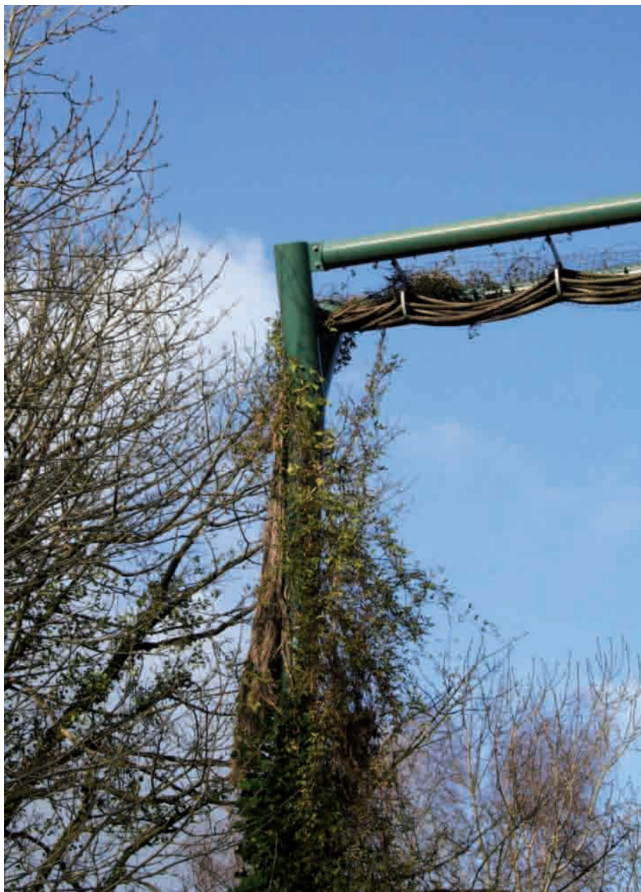
Figure 2. Detail of A4048 dormouse bridge showing climbers growing on the supporting column, connecting to natural ropes forming the bridge structure
