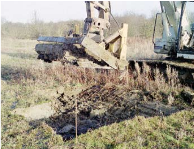
Figure 3. Donor turfs were collected using a 'fork and blade' excavator attachment specifically designed by the contractor Photo: Karl Crowther
