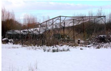
Fig. 2: Snow damage to the roof of the trap 2012
