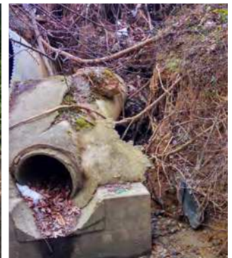
Waterways can be impacted by stormwater infrastructure that has failed
