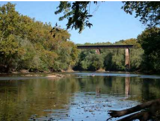
Railroad crossing over the Monocacy River, 0.5 miles north of the Potomac River
