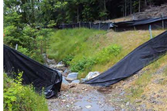
A sediment fence that has failed, allowing soil to enter the aquatic system
