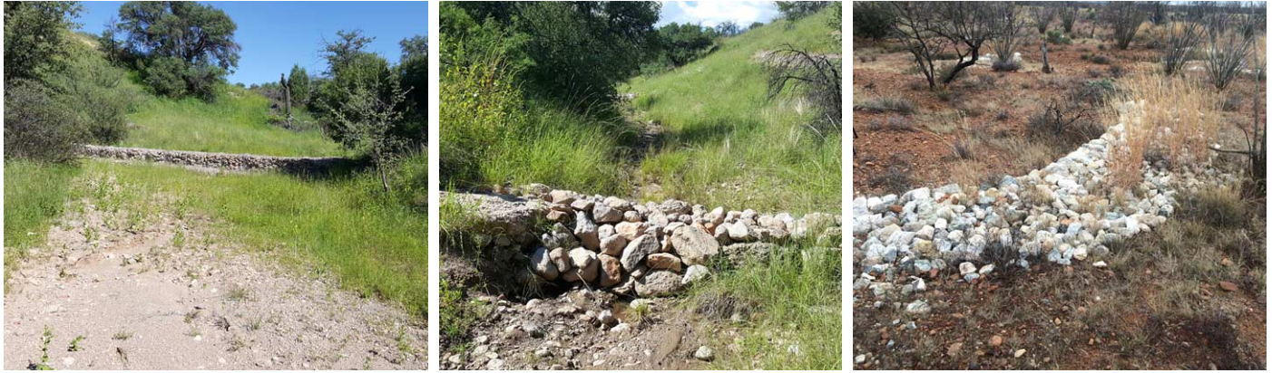
Figure 1. Watershed restoration structures (from left): Gabion, a wire enclosed rock structure in the channel; Check dam, a loose rock structure in the channel; and Media luna, a loose rock structure on the floodplain.
