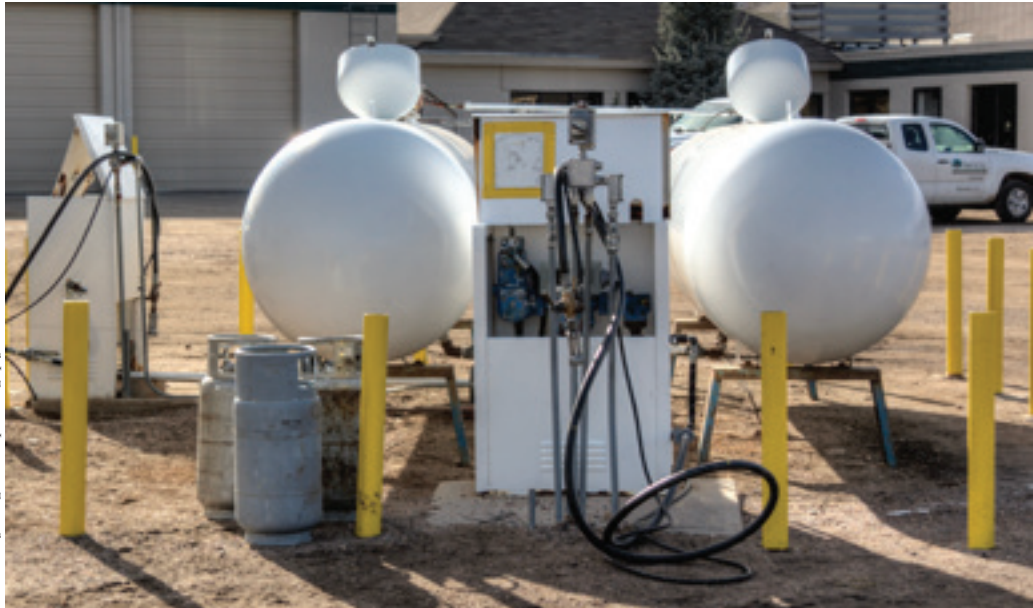
Propane tanks fuel about 25 vehicles
