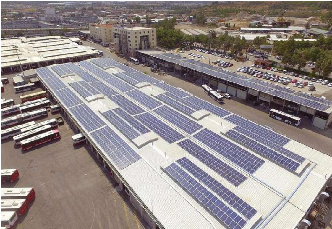
The electricity requirements of ESHOT buses will be supplied by solar generation.
