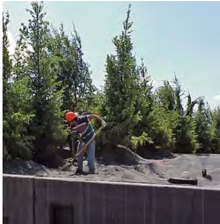
A worker shovels a shale-aggregate soil mix on the roof garden of the Latter-Day Saint’s Conference Center during its installation.
