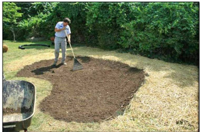
Fig. C-15. Leveling a rain garden to produce a flat bottom with sloped edges: a modified "bowl-shape" Photo by Bill Shuster, USEPA-RD
