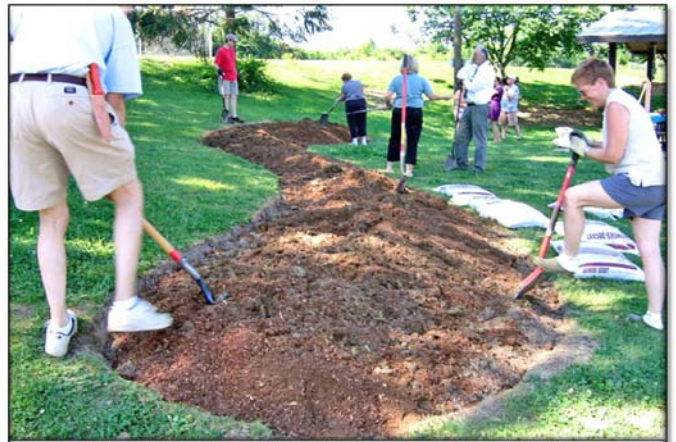
Fig. B-7: Topsoil and amendments added to raise CIP bed to 12" height Photo by Dave Dyke
