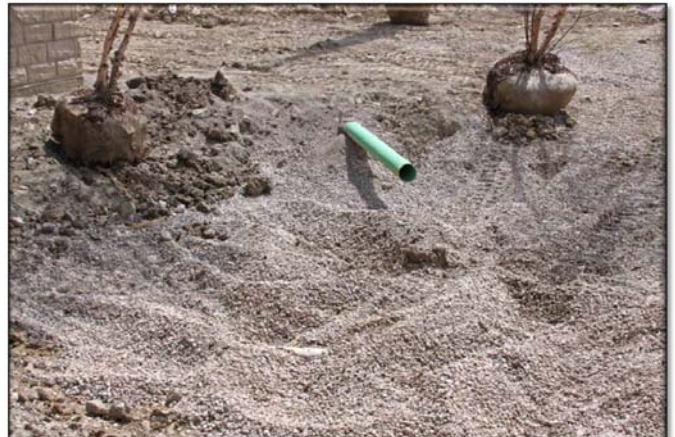
Fig. C-9: Gravel blanket being installed beneath a rain garden Photo by Joe Boggs
