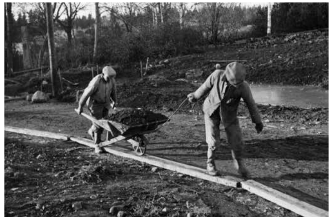
■ Fig. 4. Niagara Stream garden being dugged out in the 1940's. (Unknown photographer, NMBU Photo Archives, UMB-030784)
