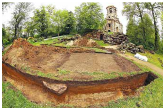
■ Fig. 4. Archaeological evaluation of the old path structure in the area of the temple of Mercury, by Achim Wendt and Claudia Binder, 2016. (From: RNZ-Archiv, Photographer: Norbert Lenhardt, 2016)
