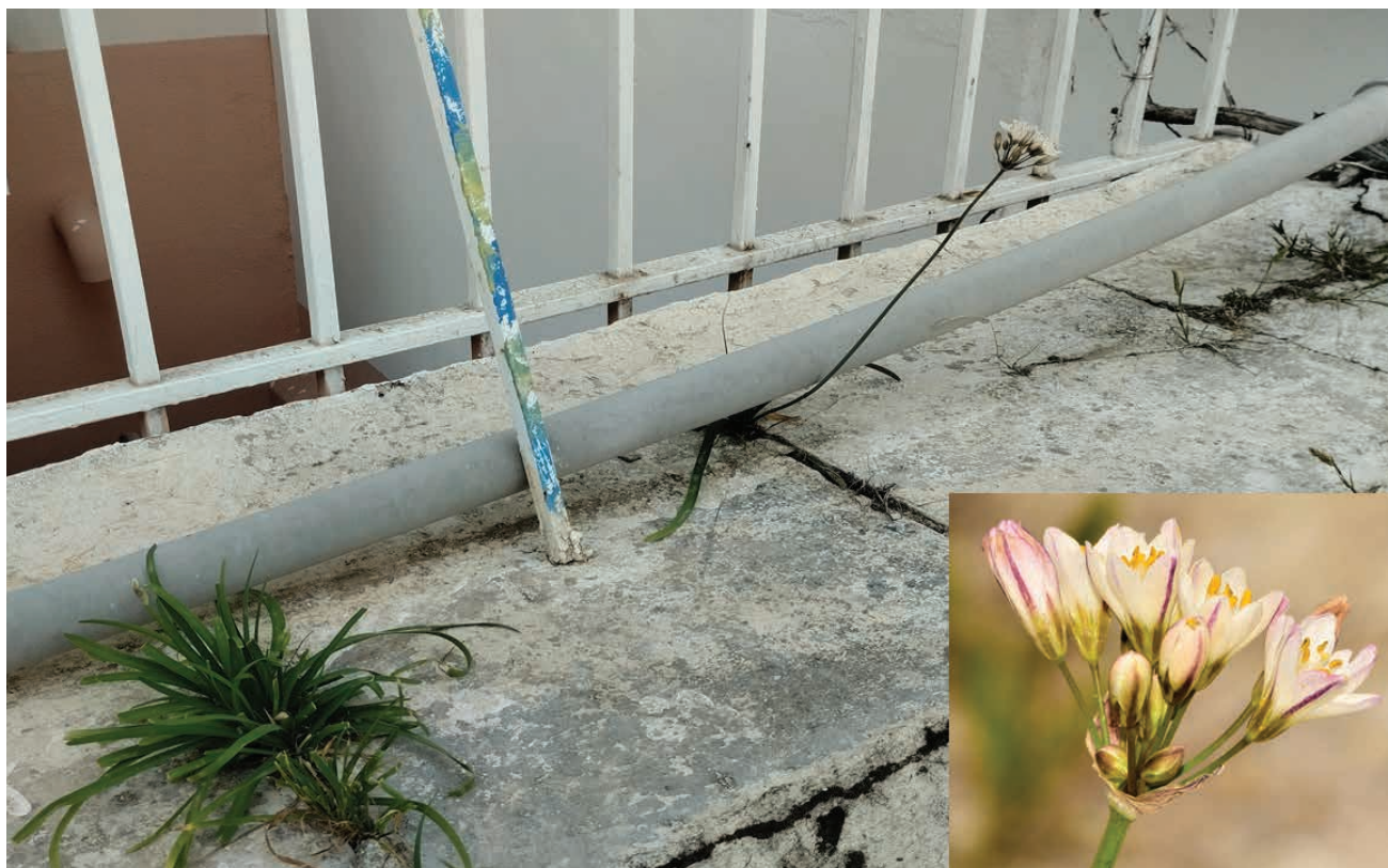
Fig. 28. Nothoscordum gracile in concrete cracks of roof terrace (photo G. Kofinas).
