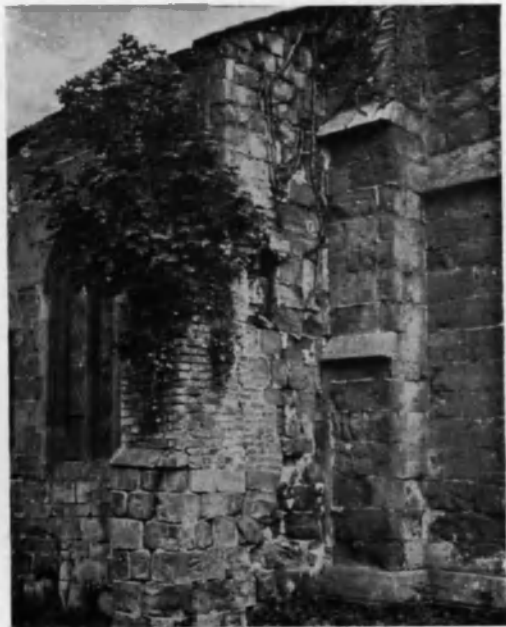
MALTBY CHURCH, LINCS., 1940. Before Repair in 1940.
