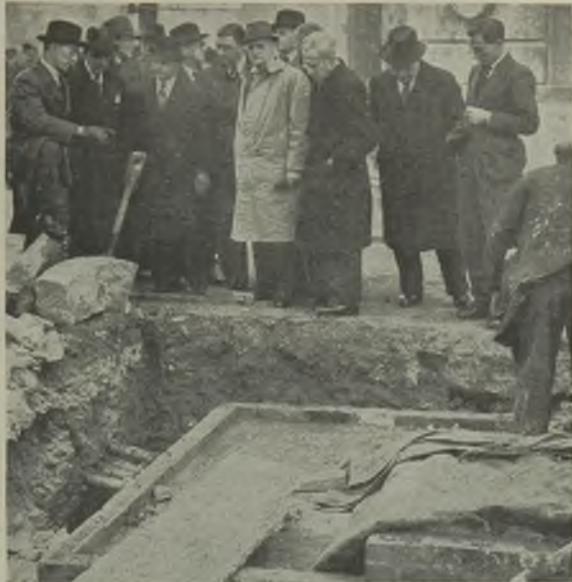
Mr. R. G. Widgery, borough electrical engineer of Dover, describing damage caused by a shell to an underground substation now being repaired
